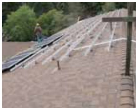
Solar installation at St. John's Episcopal, Oakland
